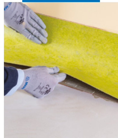
Installation of cove-base and laying of s covers with Ultrabond Eco Fast Track
